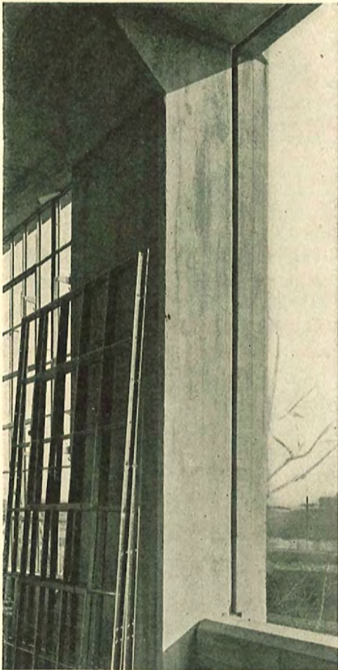
Groove provided in concrete walls to receive flange of Lupton Pivoted Windows.
