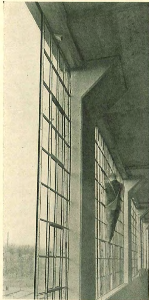
Lupton Pivoted Windows in concrete walls. Windows are plumbed, wedged and then grouted.
